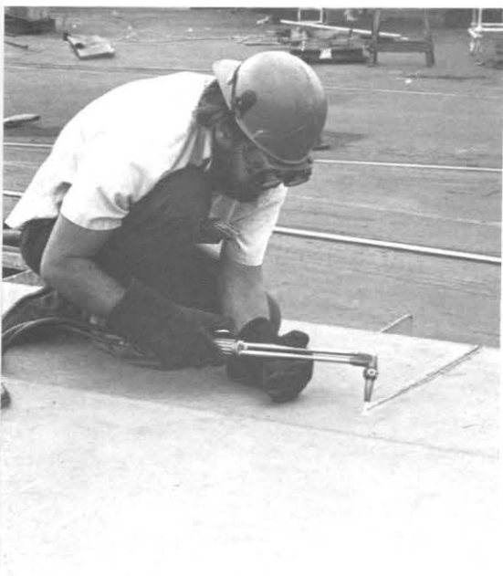
A burner cuts a steel plate. This piece will then be welded to other plates to form a subassembly of a larger module.
